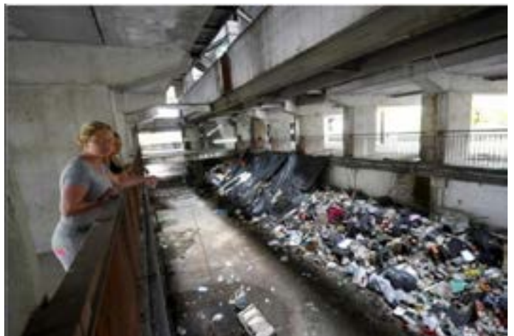
Fig 10. Rubbish at base of void
